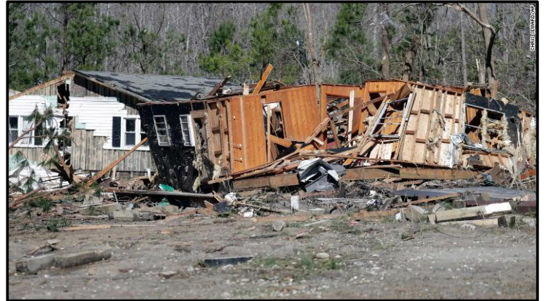
Homes were heavily damaged near Sunset Beach, NC, after the overnight storm.
