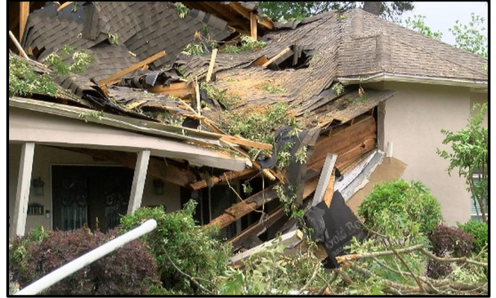
Tornado damage extensive in Jackson, MS neighborhoods.
